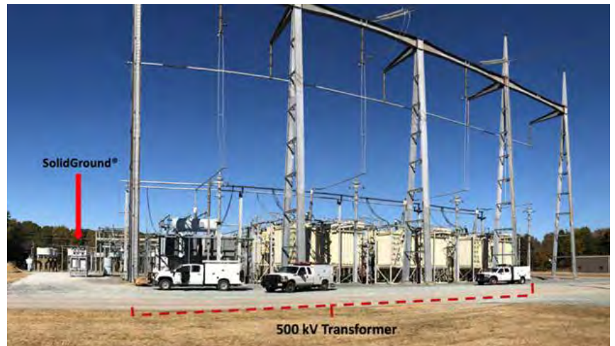
“SolidGround” NBD protecting a 500 kV transformer in the TVA grid. This transformer would cost upwards of $20 million, and years to replace if it were destroyed by ground induced currents from solar weather. The “SolidGround” unit protecting this transformer costs approximately $500k, or 2.5% of the value of the total asset.
