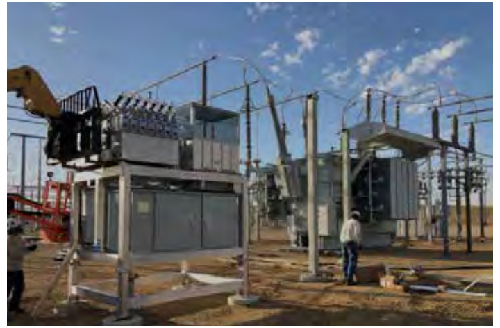
"SolidGround" NBD protecting DOE's 345 kV transformer in the WAPA grid in South Dakota.
