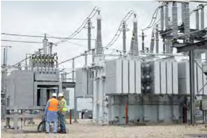
"SolidGround" on 345KV transformer in the ATC grid in Wisconsin (9+ years of testing)
