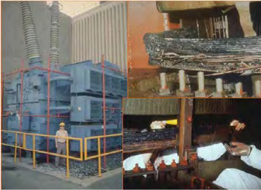
This transformer sustained major damage from GICs induced by the March 1989 Solar Storm. Photo credit: Dr. Jeffrey J. Love, USGS
