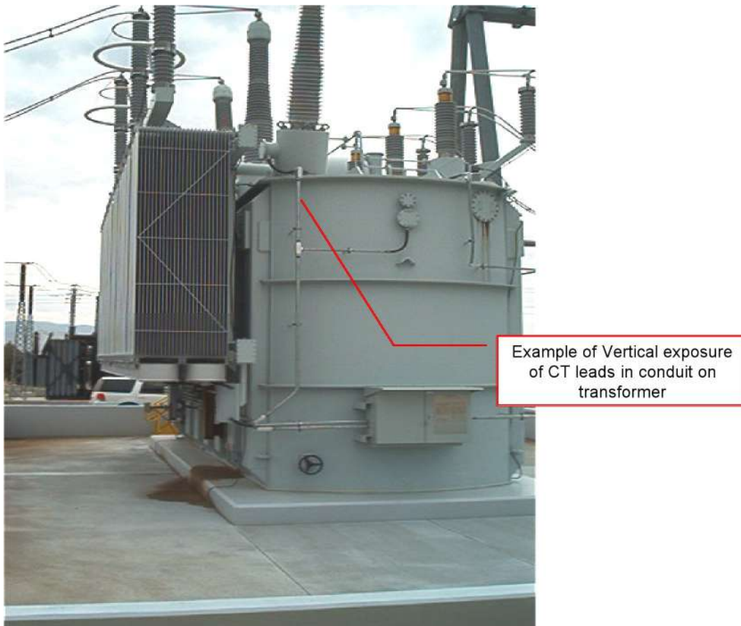
Figure 7-18. Exposure of cable conduits on transformers.
