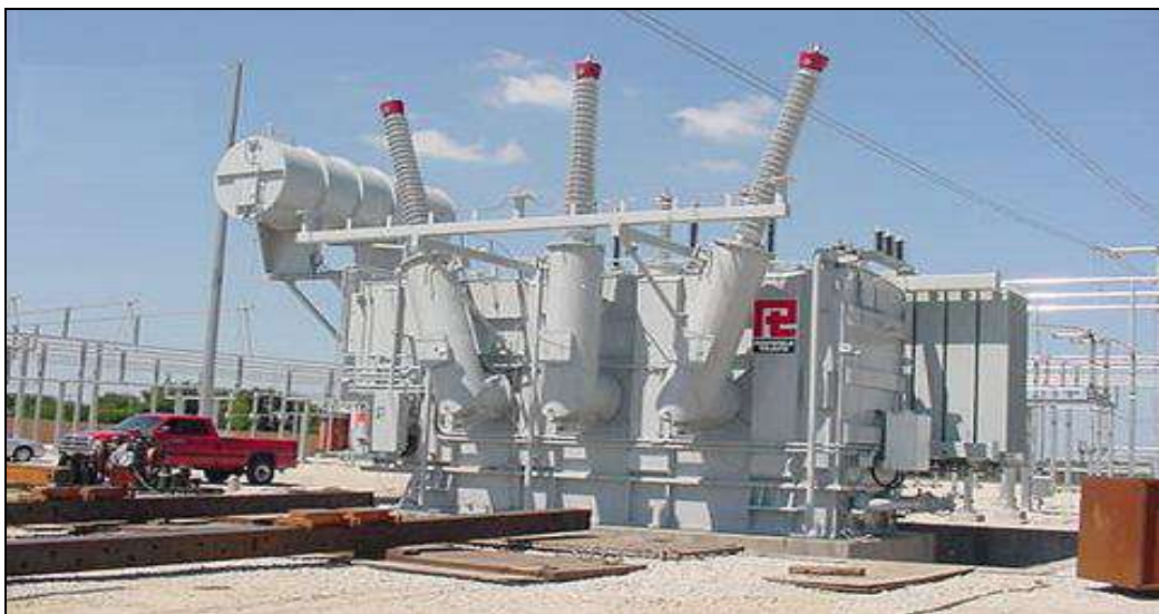
Figure 3. Installation of a 345 kV Transformer
