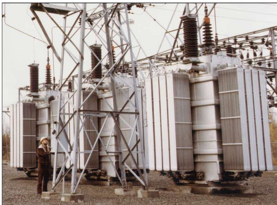
Figure 2: Large Power Transformers
