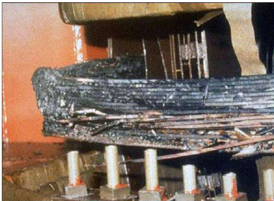
Figure 3: Damaged Transformer Winding Attributed to an Electromagnetic Event
