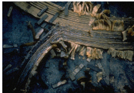
Figure 2-3. GIC Damage to Transformer During 1989 Geomagnetic Storm
